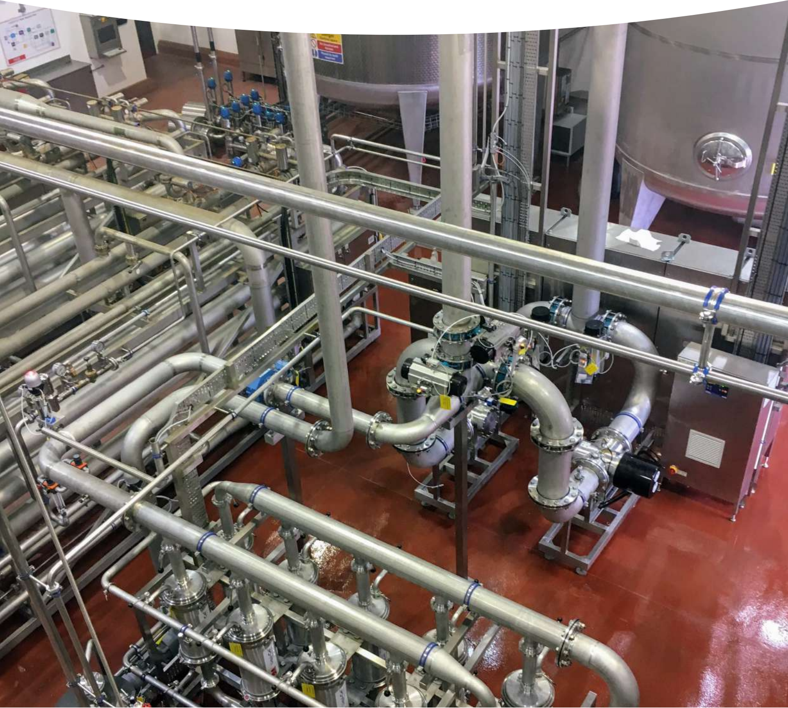
Stainless steel pipework part of the process water treatment plant
