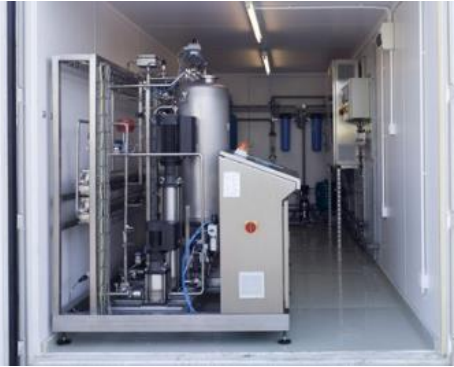
Containerized CDI System
