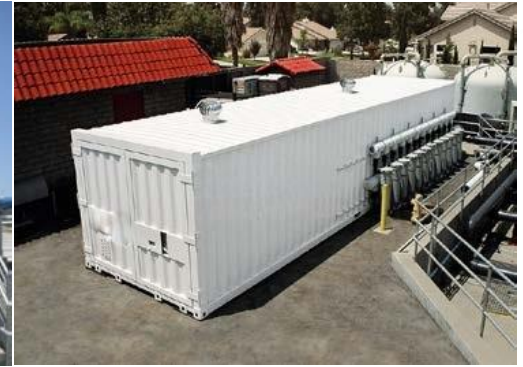
Containerized IX Unit
