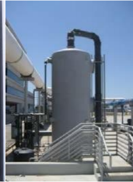
Biotrickling Filter Tower
