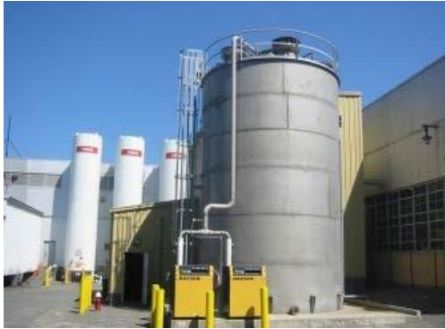
MBR – Beverage Plant
