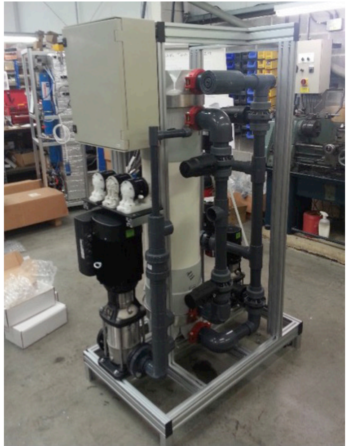
Single Ultra Filtration (UF) rig used for the on-site trial
