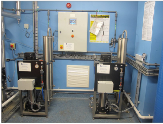
The duplex duty standby RO system at Guy's Hospital
